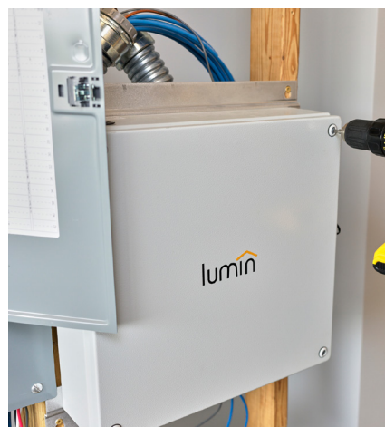
Smart breaker boxes, like the hardware-agnostic Lumin Smart Panel shown here, turn standard panels into smart panels by providing comprehensive energy control and extending whole-home backup.
